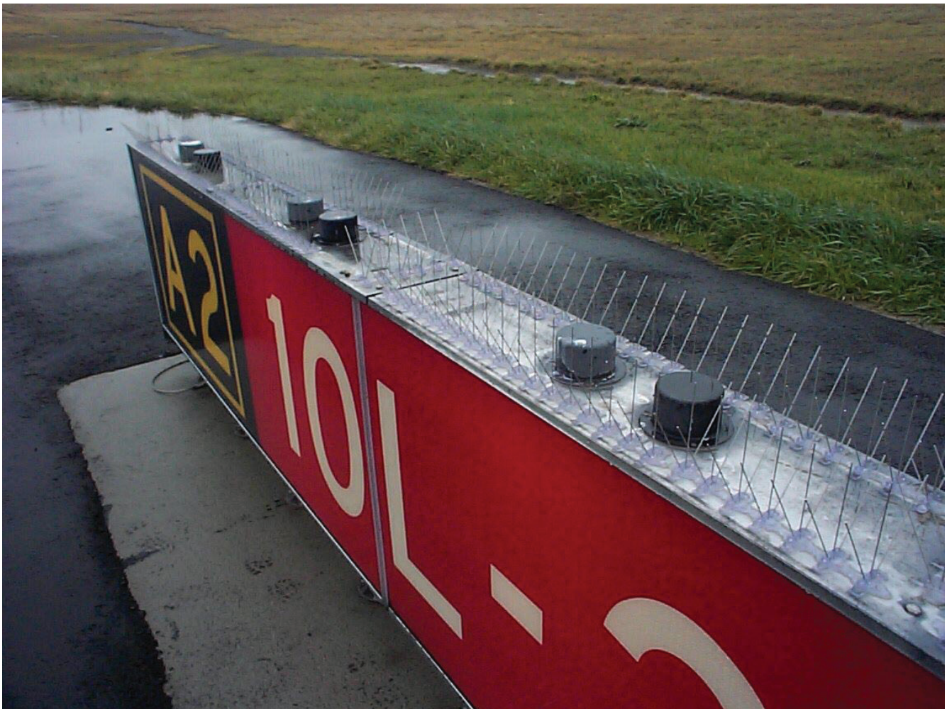
FIGURE 11 Antiperching devices used to deter birds from a low level windshear alert system (Source: Steve Osmek).
