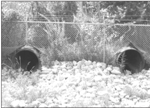
FIGURE 1. Culverts through a fence line can create large passageways for wildlife at airports. (Photo by J. E. Kubel)
