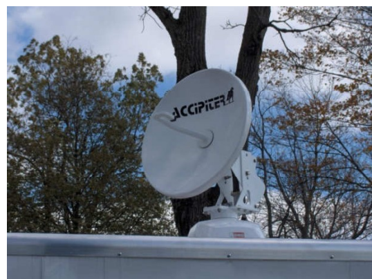
Figure 5: Avian radar dish antenna.
